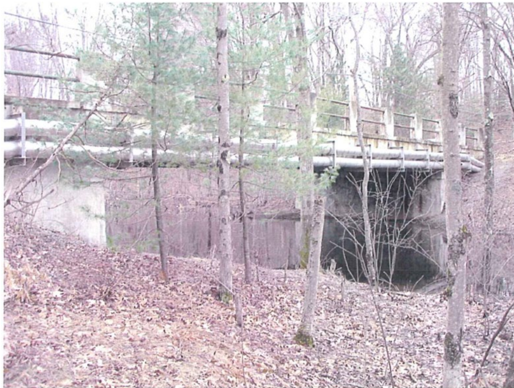
Photograph No. 6: Lowell Road (MM 2.611) is overtopped by approximately 1-foot during the hypothetical storm-day dam failure
