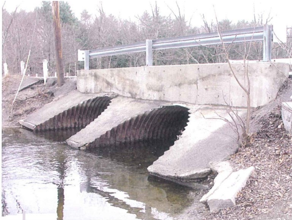
Photograph No. 5: Shaker Road (MM 1.987) is overtopped by approximately 6-feet during the hypothetical storm-day dam failure.
