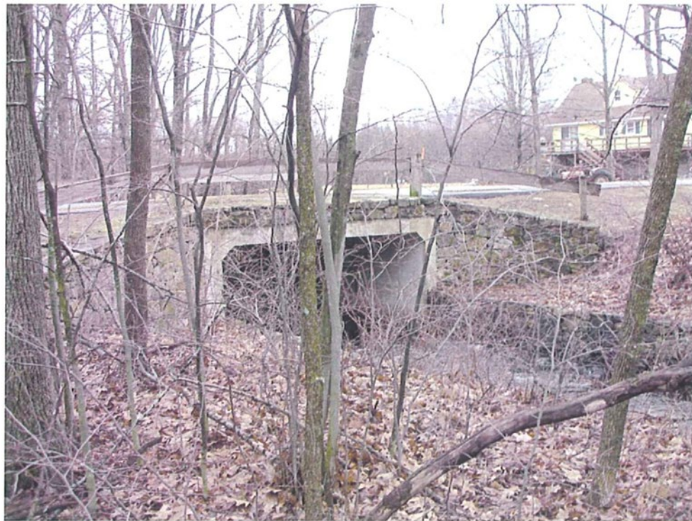
Photograph No.2: Brook Trail Road (MM 0362) is overtopped by approximately 6-feet during the hypothetical storm-day dam failure
