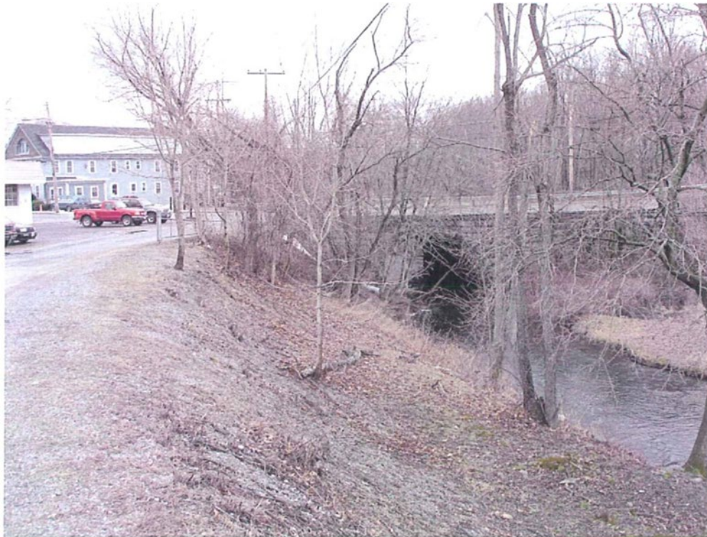
Photograph No.4: Leominster Road (MM 1383) is overtopped by approximately 5-foot during the hypothetical storm-day dam failure.
