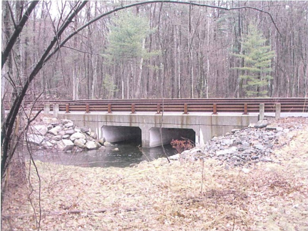
Photograph No.1: Catacunemaug Road (MM 0.682) is overtopped by approximately 7-feet during the hypothetical storm-day dam failure
